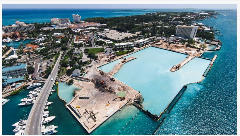
Hurricane Hole Superyacht Marina at Paradise Landing aerial view of construction progress
