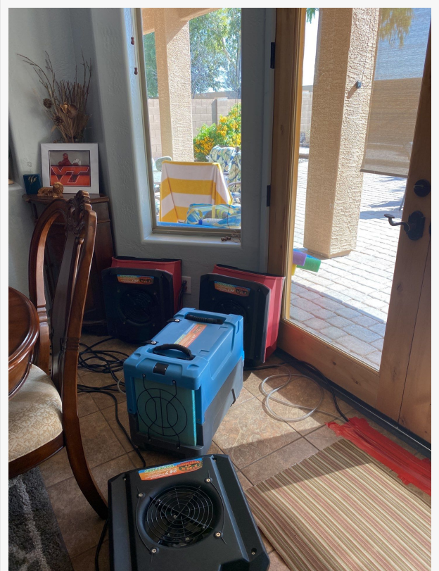
Water Damage equipment that is circulating the air and removing moisture to expedite the dry out process.
