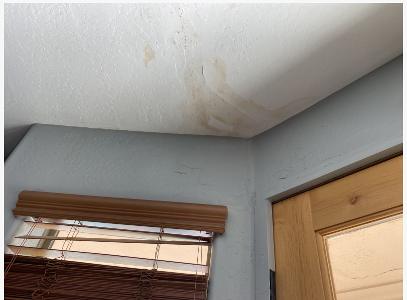
Visible signs of water damage from a leak in the ceiling.
