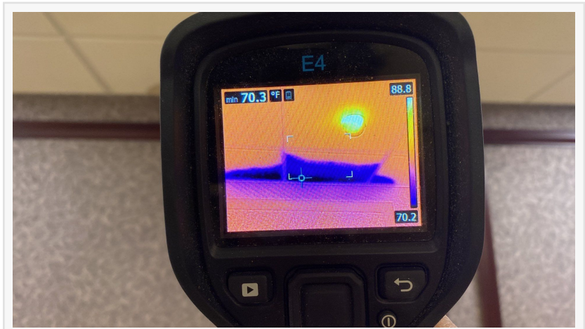
Thermal Imaging of water damage in ceiling tiles.
