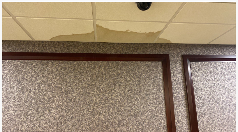
Visible water damage in ceiling tiles.
