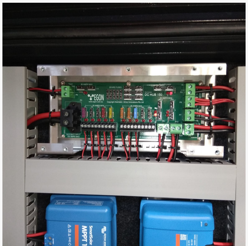
Egon DC-Hub installation 1
