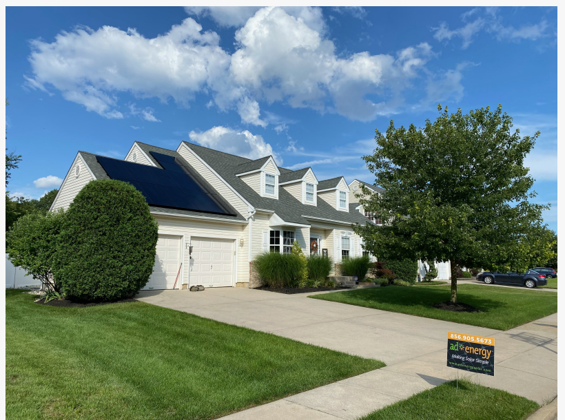
Ad Energy Solar Installation
