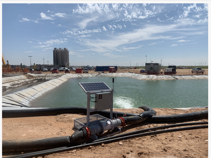
Flow-Sync automation skid boosts productivity in fracking water supply by more than 50 percent
