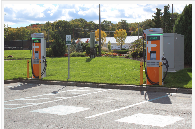
Two new DC Fast Chargers (DCFC) installed at Bally's Twin River by Inovis Energy
