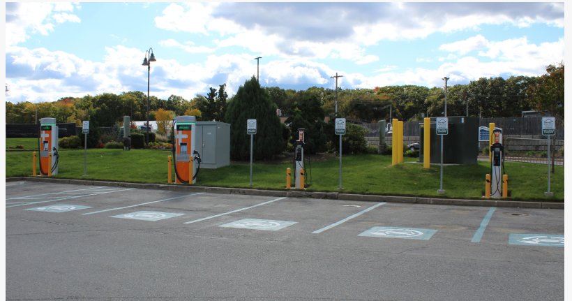
Bally's Twin River North Lot Charging Stations by Inovis Energy
