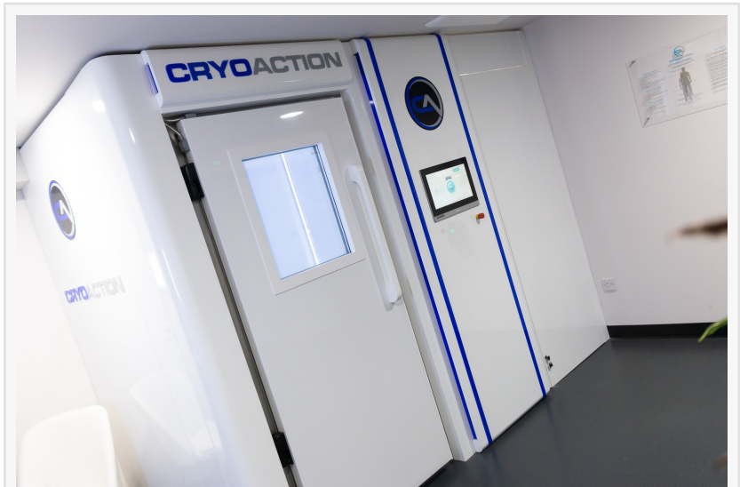
Cryotherapy chamber installed in Aesthetics Ayrshire - Photo by Aesthetics Ayrshire
