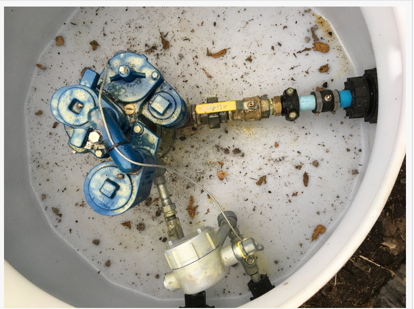
Newly installed ethanol pump, treated with HinderRUST HV100, January 2020.
