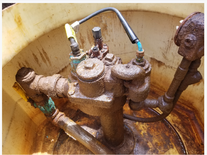
Untreated, rusted underground containment center.
