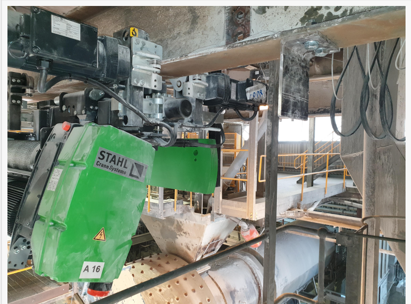
Stahl 5t swl Electric Wire Rope Hoist Installed at a UK Cement Work
