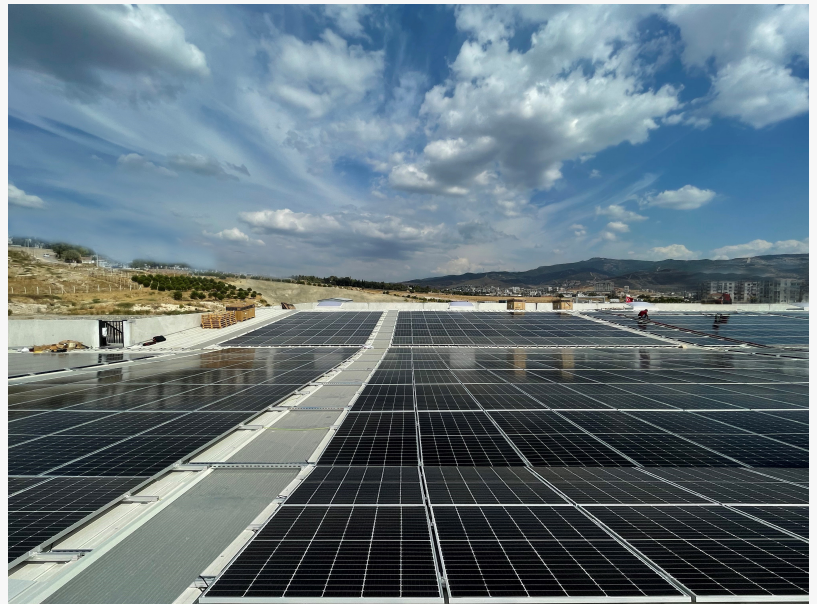
solar power plants
