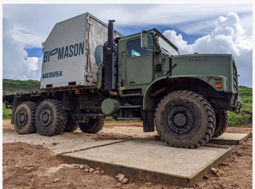
Biomason's MEDUSA team successfully grew a bioconcrete slab during an inter-military exercise in the South Pacific in July 2021.
