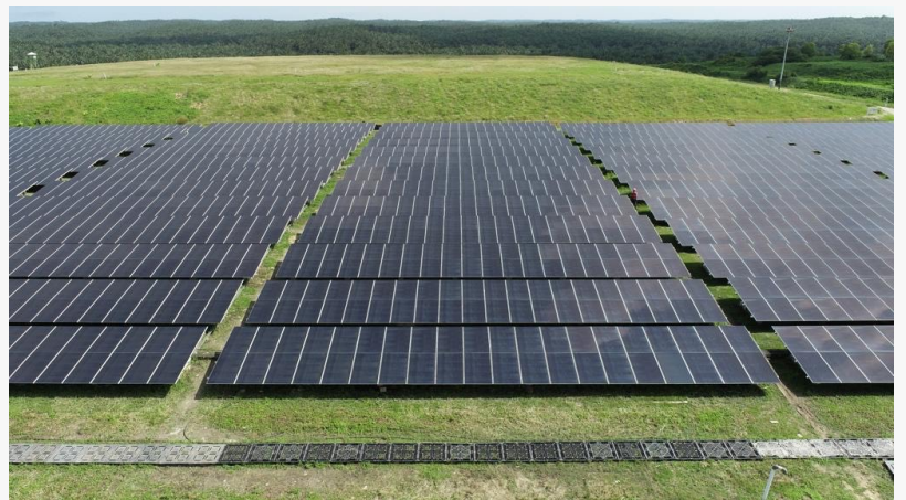
Solar panel project with the commissioning of a 1-megawatt solar panel at the APRIL operational site in Riau province, in Sumatra, Indonesia.
