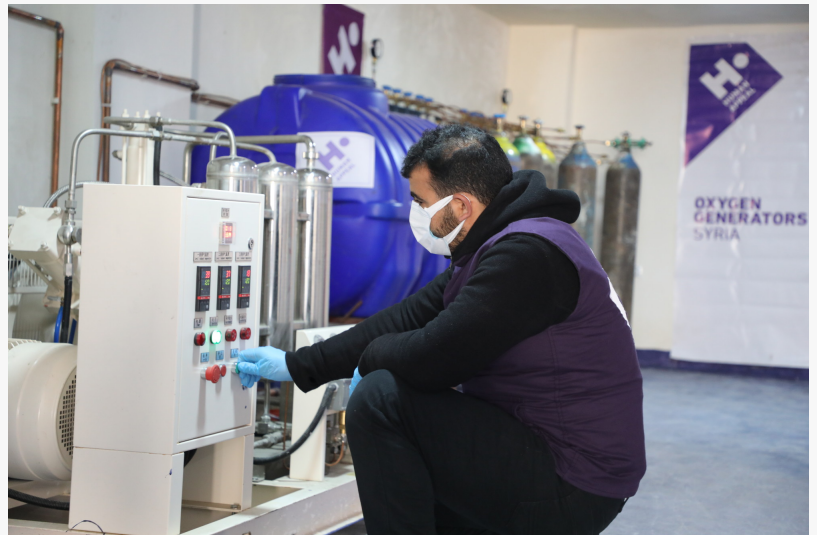
Oxygen generators installed by Human Appeal in Northern Syria
