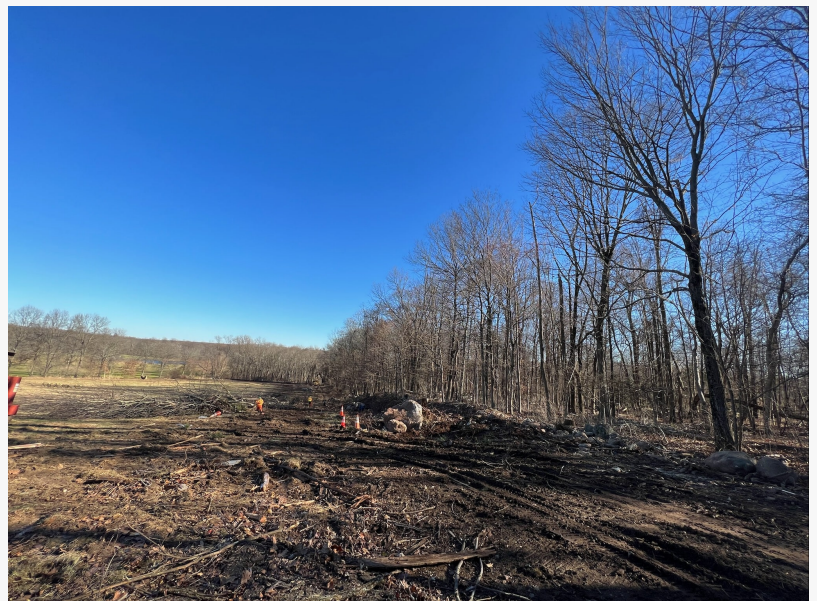
Crews remove old driving range netting system and clear worksite for new netting system.
