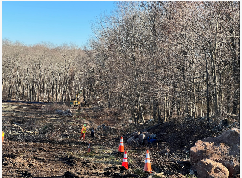
Crews remove old driving range netting system and clear worksite for a new netting system.
