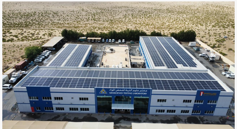
Sharaf DG Energy has completed the installation of 950 solar panels which are now helping Geoscience Testing Lab generate 723,500 kilowatt-hours of electricity annually
