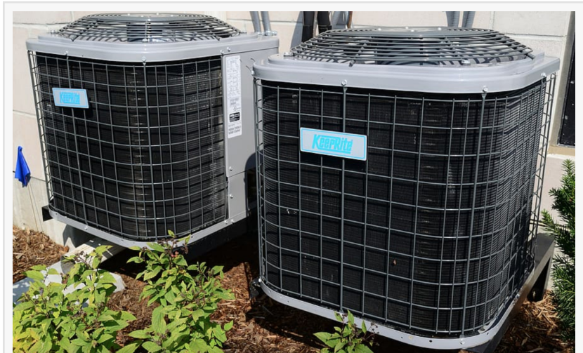
Cooling System Heat Pump Inspection in Phoenix Arizona
