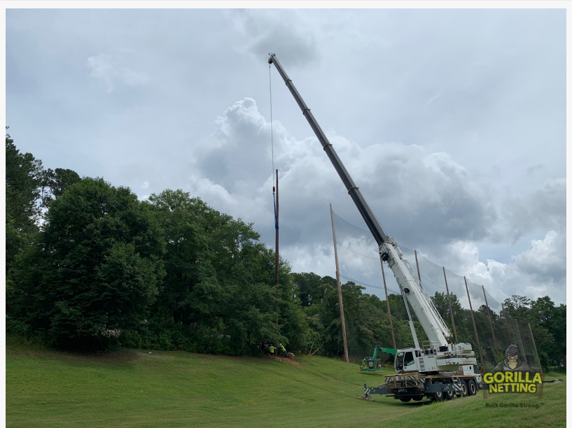
Gorilla Netting installation crew install 90-foot tall pole to extend driving range netting system at The First Tee of Atlanta.
