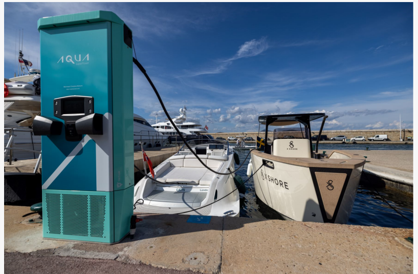
The Aqua 75 dual CCS configuration supercharging 2 electric boats simultaneously (Credit Aqua superPower Ltd)
