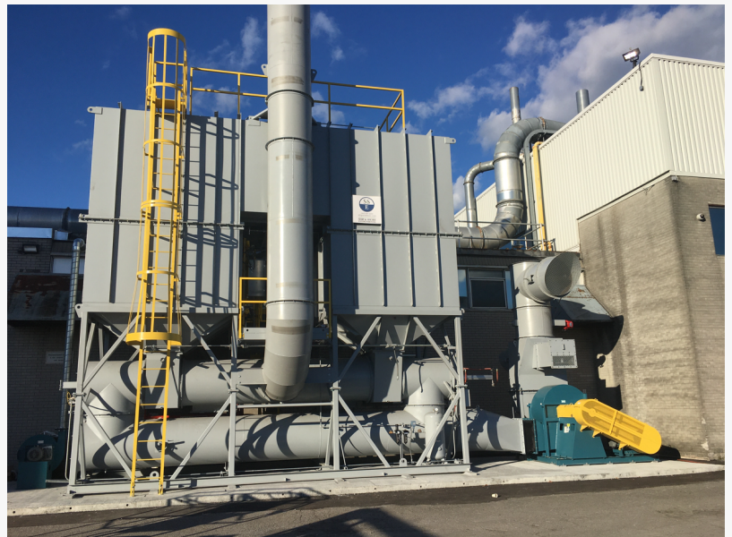
Ship & Shore RTO Installation – Cleaning the Earth One System at a Time
