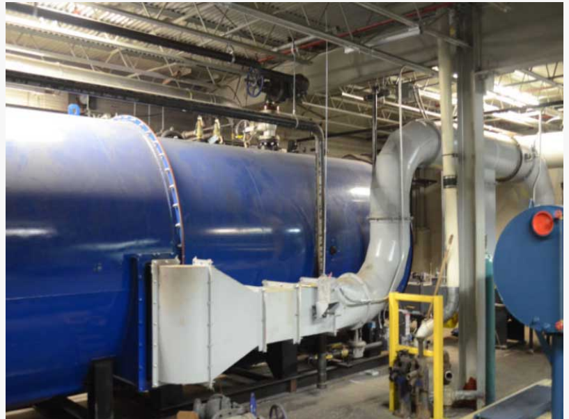
Ship & Shore Environmental's Steam Generating Thermal Oxidizer (SGTO)
