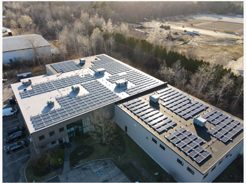
Cirrus LED Solar Rooftop Panel Array
