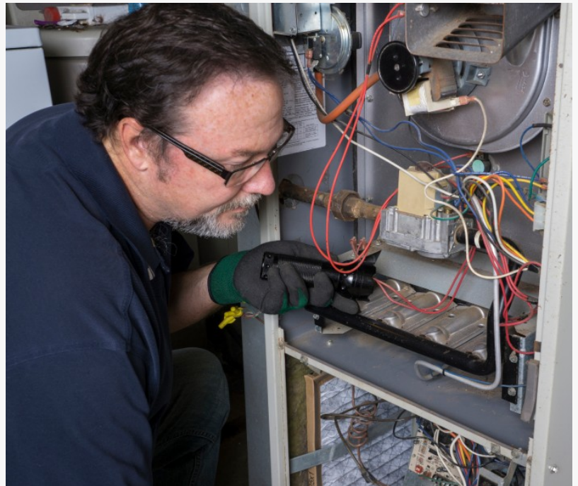
HVAC maintenance in Garland
