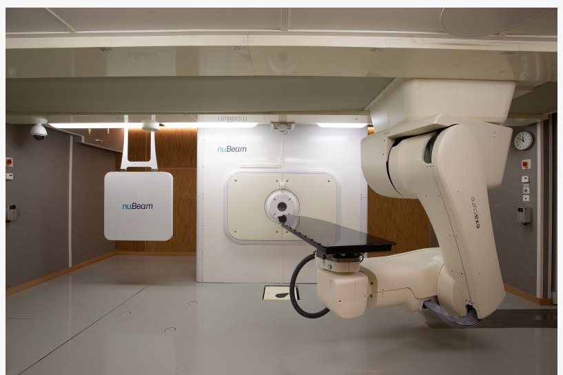
The nuBeam® treatment room showing shutter, beam-shaping assembly and positioning robot
