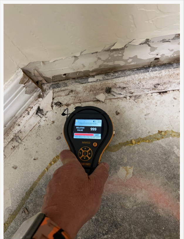
Moisture Meter showing that the subfloor is wet .
