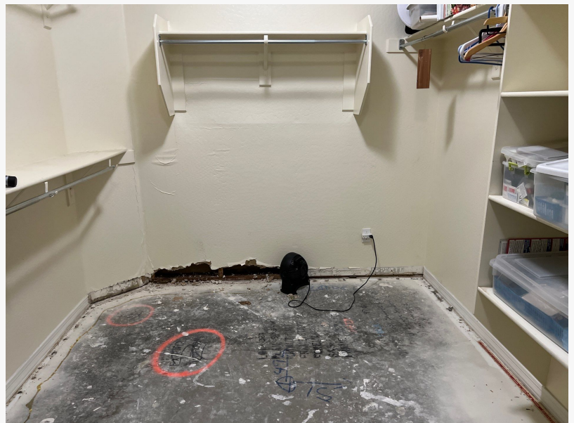
Visible signs of water damage in a walk in closet.
