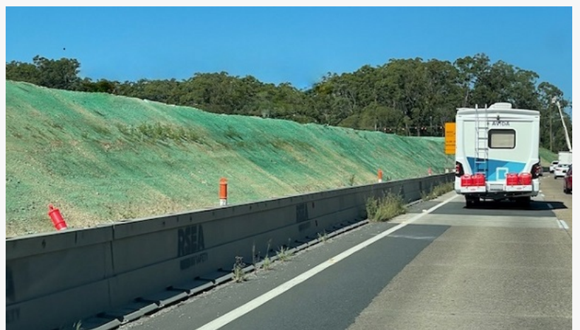
RST Solutions' soil binder Total Ground Control applied to an embankment is reducing dust and erosion during major roadworks
