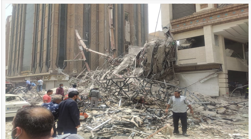
A large portion of the Metropol tower in Abadan, southwest Iran, collapsed Monday morning local time leaving at least seven dead and 31 injured. State media are reporting there is a possibility of more than 50 to 80 others being trapped under the rubble.
