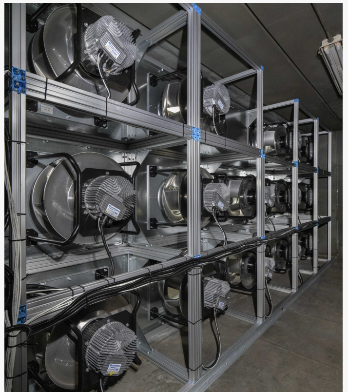
New Fan Arrays in Neptune, NJ facility
