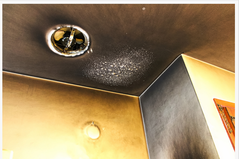
Fire Damage in Dayton Ohio
