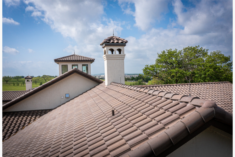
Key's custom home design/build in Denton, TX. - Protected with a lightning protection system.
