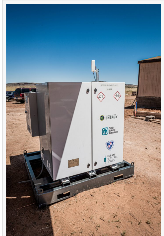
Urban Electric Power's 13 kilowatt-hour battery can supply electricity for several days when necessary between recharges by solar panels. The system replaces lead-acid batteries formerly used. Credit: Umer Anwer, Urban Electric Power
