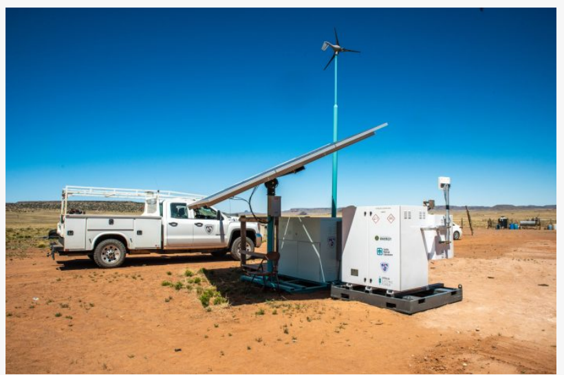
New Urban Electric Power rechargeable alkaline battery system with recharging solar panel, on the Navajo Nation near Dilkon, Arizona. The safe, affordable system brings energy equity to families living off-the-grid. Credit: Umer Anwer, Urban Electric Power
