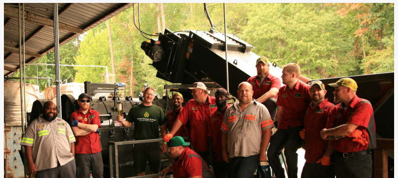
BioJoe Renwick, third from left, and his crew at Green Energy Biofuel commission their newly installed depackaging equipment, which can process industrial bulk and palletted prepackaged foods.
