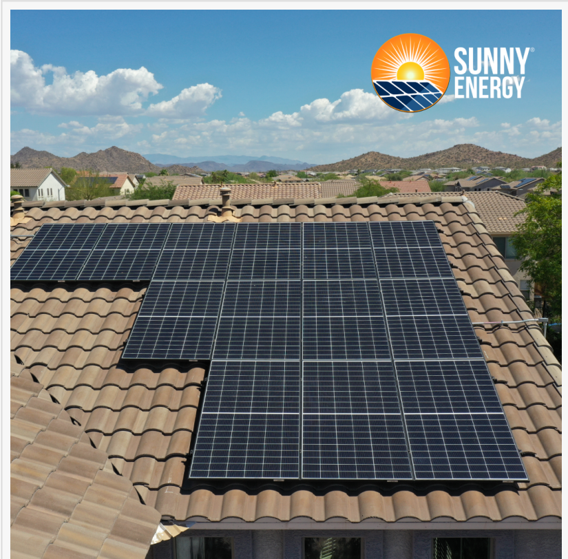
Sunny Energy Solar Installation In Phoenix
