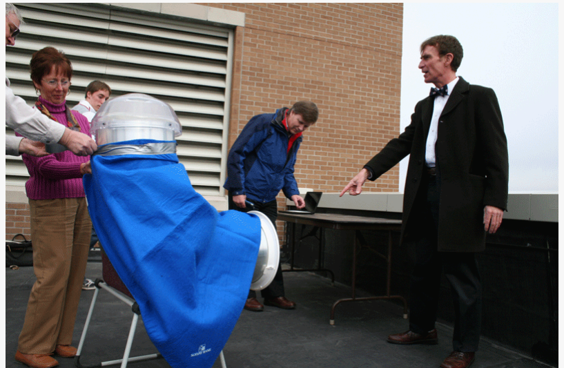
Bill Nye and team get the Solatube Tubular Daylighting Device ready for install
