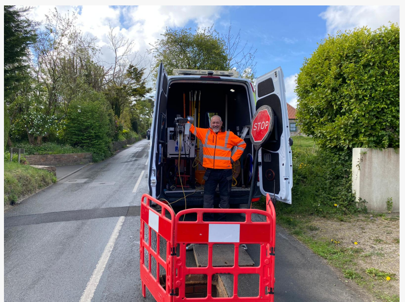
Chris Chesworth, Electro Scan (UK) Ltd. at work in Jersey, Channel Islands.
