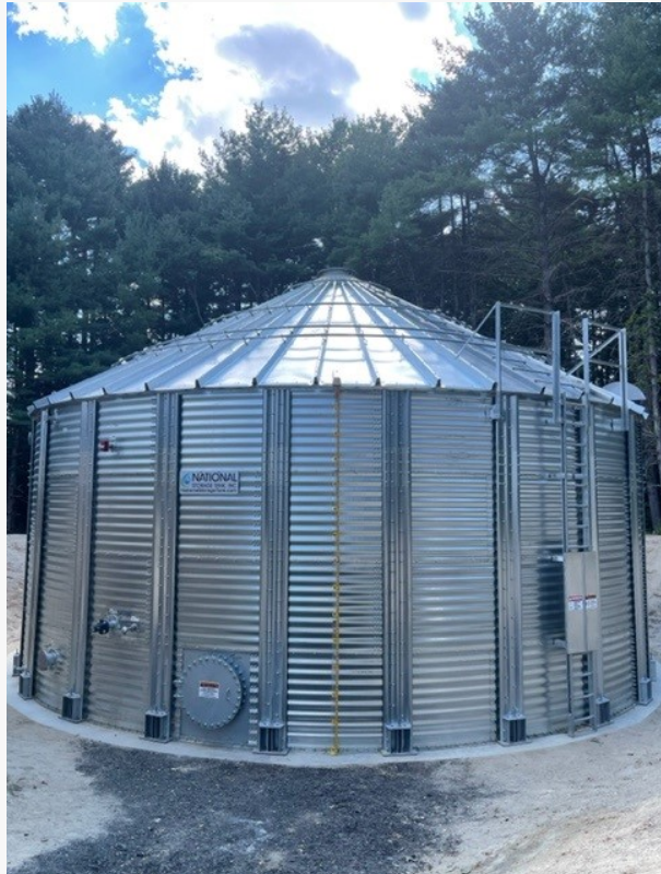
Fire protection tanks to 6-million gallons
