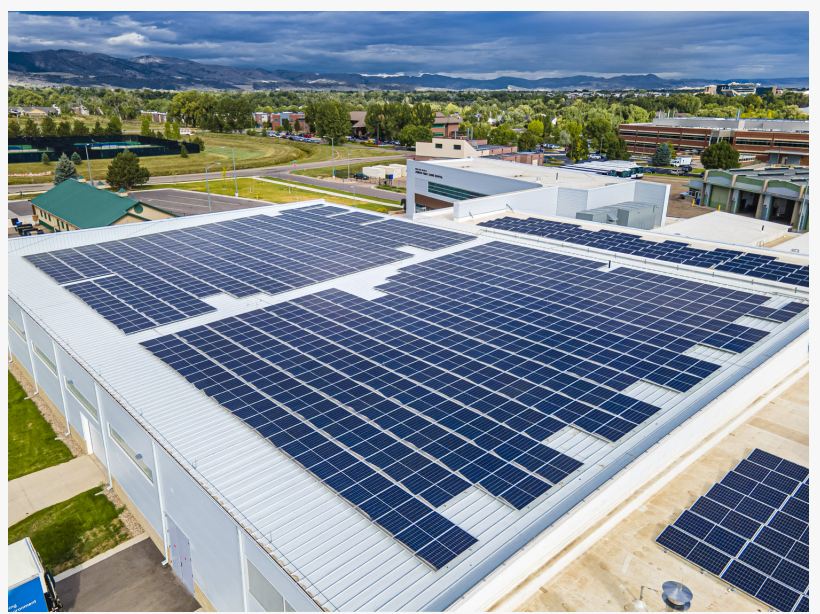
Johnson Family Equine Hospital at Colorado State University in Fort Collins Colorado - photo credit Namaste Solar
