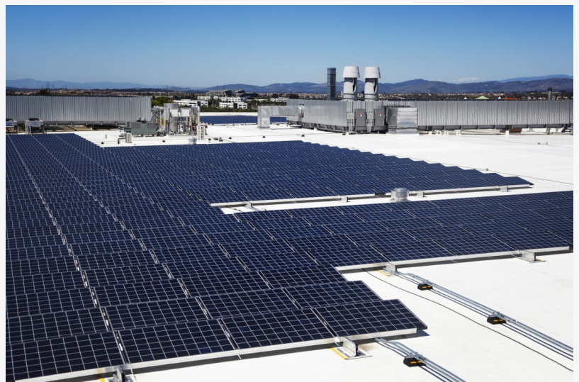
Alfa Group has installed solar panels, geothermal heating systems in many of its office buildings, logistics areas and commercial buildings already for the past decade
