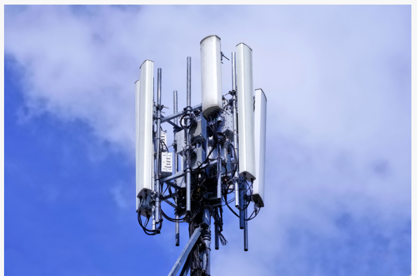
5G Base Station
