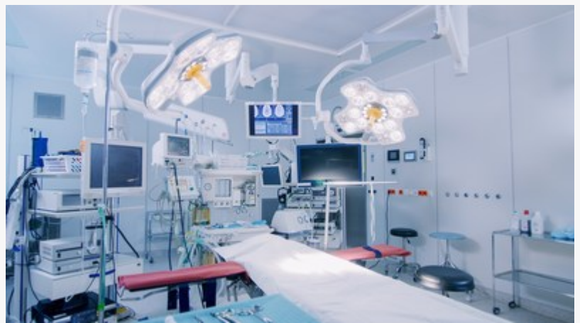
Operating Room Integration
