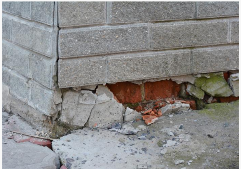
home requires foundation repair due to crumbling exterior wall
