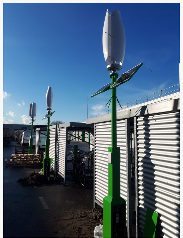
Wind and Solar E-bike Charging Poles
