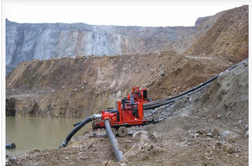
Dewatering Pumps Industry
