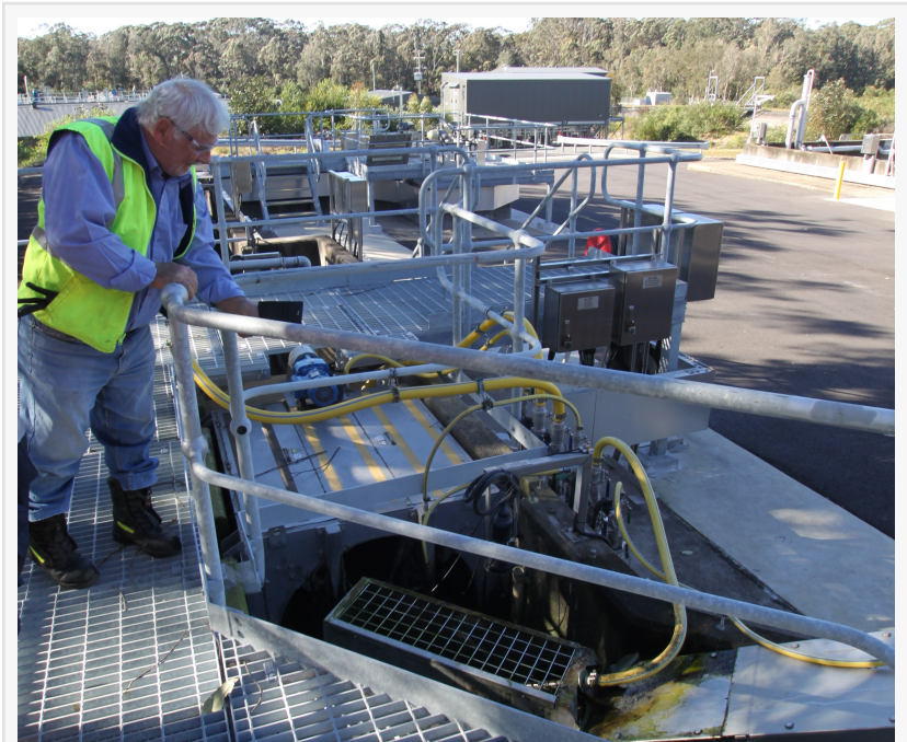
A technician inspects the smoothly functioning new locally manufactured Rotary drum screen and compactor from CST Wastewater Solutions.
