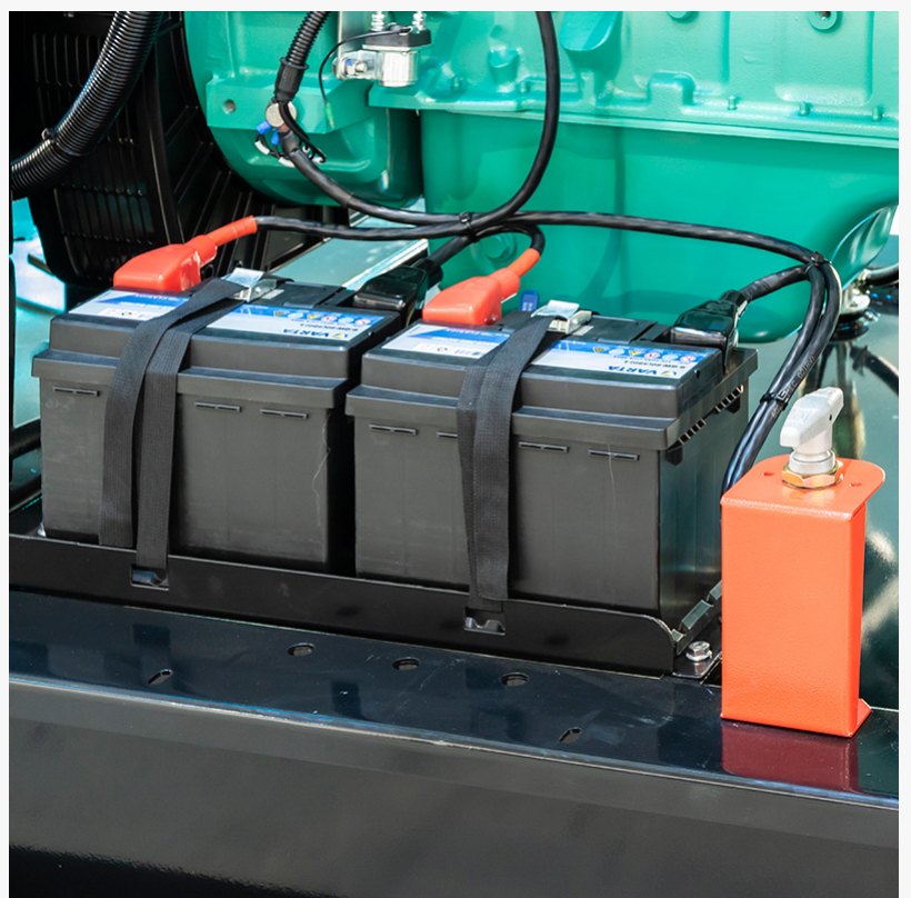
Genset Battery Market
