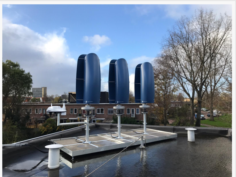
Three installed small size Wind Tulips
