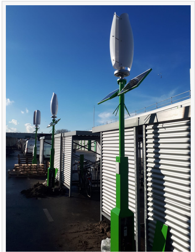
Wind and Solar E-bike Charging Poles
