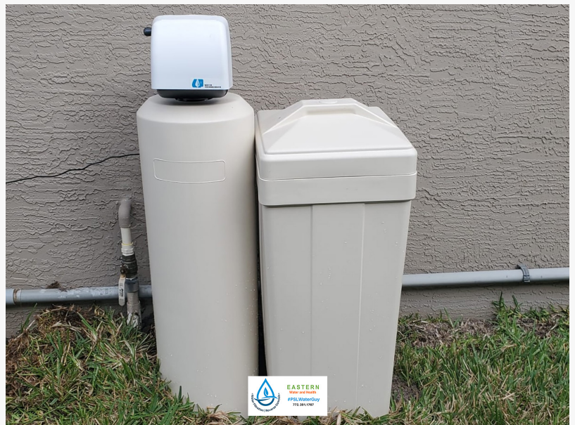
Eastern Water and Health - Water Softener Installation
