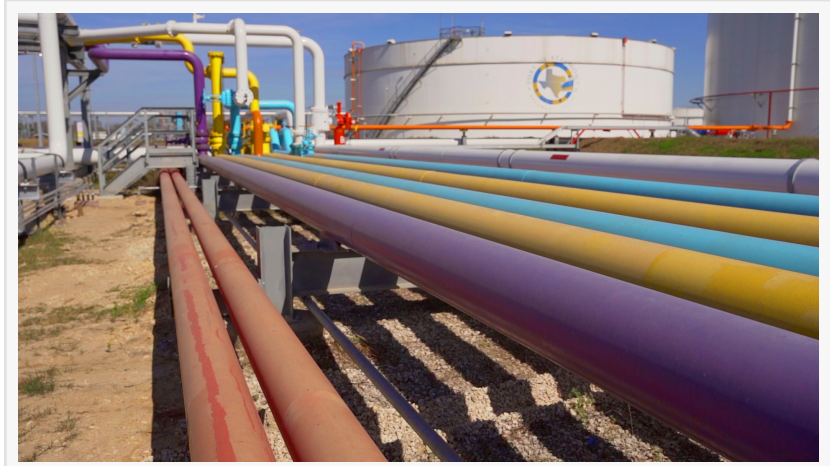
Cross Channel Pipelines, Jefferson Energy Terminal
