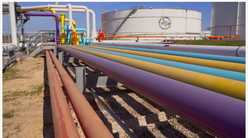
Cross Channel Pipelines, Jefferson Energy Terminal
