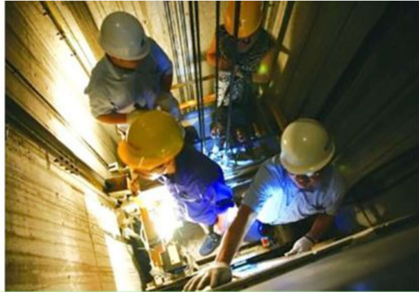
Elevator Inspection Service
